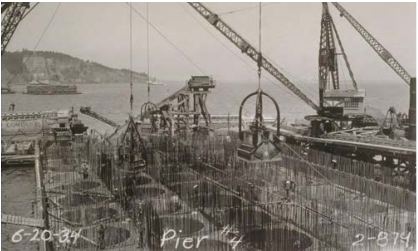
Figure 78. Excavation of central anchorage caissons on the western span of the San Francisco–Oakland Bay Bridge (Bancroft Library Collection).
