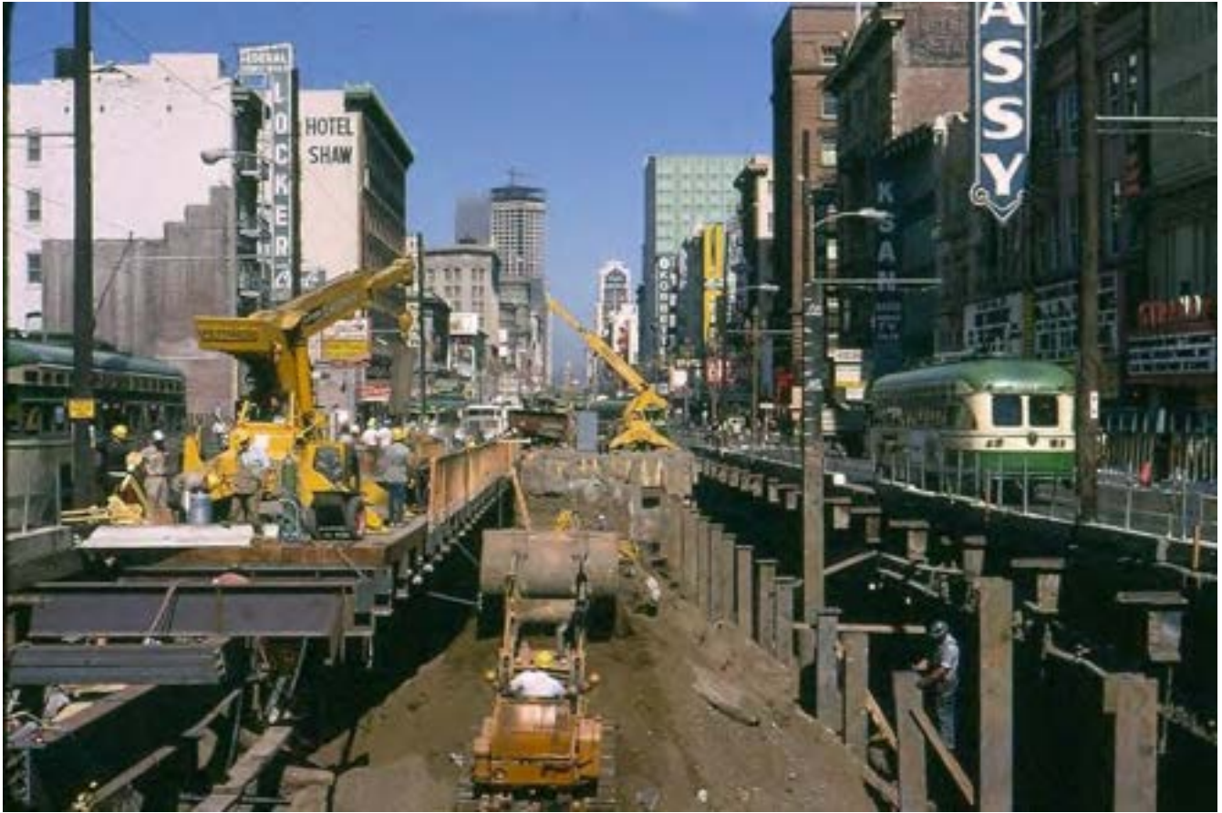
Figure 93. Construction of BART and Muni subways 1970: Civic Center Station, Market Street looking northeast (Photo from Market Street Railway, www.streetcar.org ).
