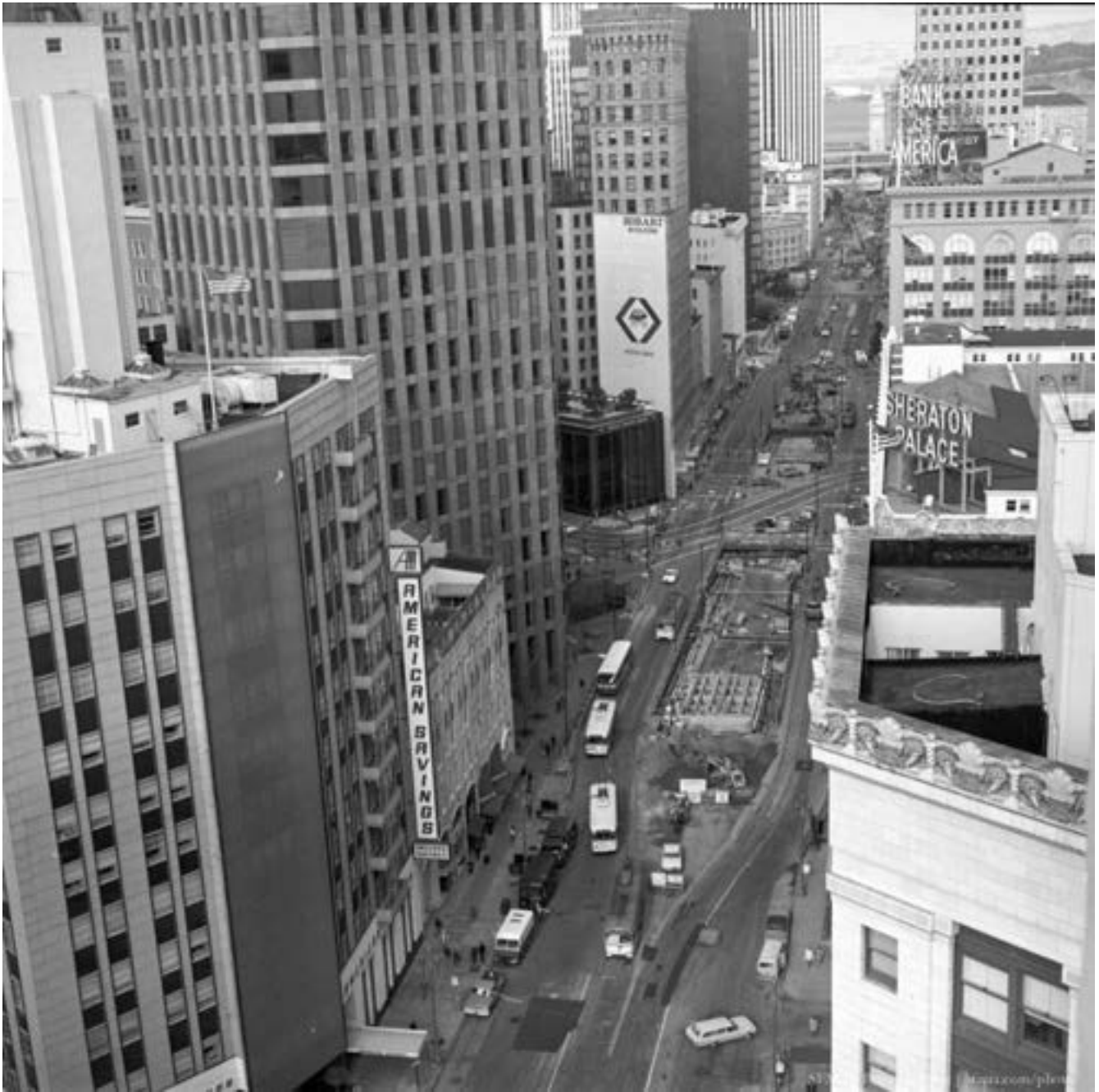
Figure 92. Construction of BART and Muni subways in 1970: Montgomery Street Station, Market Street looking northeast (Photo from SFMTA).
